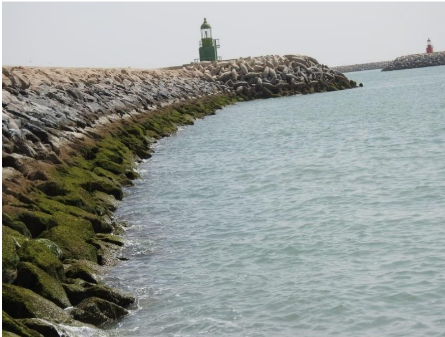
Figure 1: The eastern breakwater of Al-Faw Grand Port. Photograph by Hanaa H. Mohammed.
